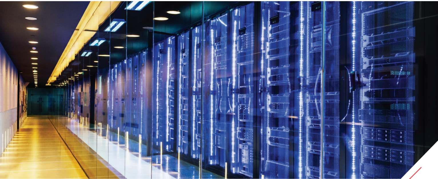
Data centers are constantly evolving and adapting to support more efficient operations; and there is no end in sight.
