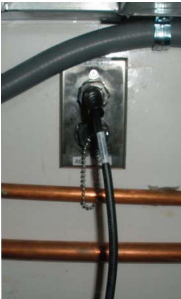
Siemon Ruggedized Z-MAX Category 6A shielded IP66/IP67-rated outlets and cords were deployed at Dodger Stadium's outdoor concession stands and kiosks
