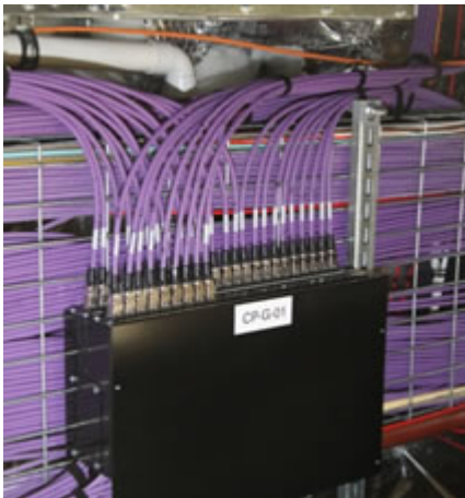
Zone Box consisting of two flat Siemon TERA MAX panels with Category 7A TERA® connectors mounted in a custom-designed enclosure under the cable tray
