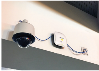
Image 2: Photo taken at a major international airport – Anyone could jump up and pull out the patch cord to the surveillance camera and wireless access point
